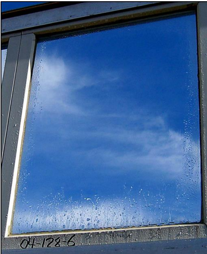
Fig CG04-06 Silicone glazing residue causing picture framing (beading of the water due to silicone residue)
